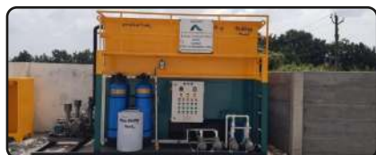
Moving Bed Biofilm Reactor Plant (MBBR)
