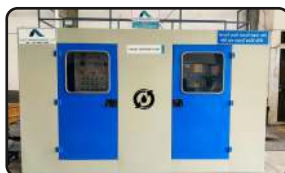
Membrane Bioreactor Plant (MBR)
