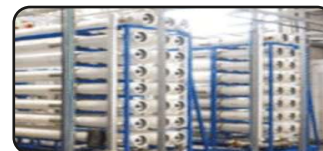
Mix Bed and DM Plant
