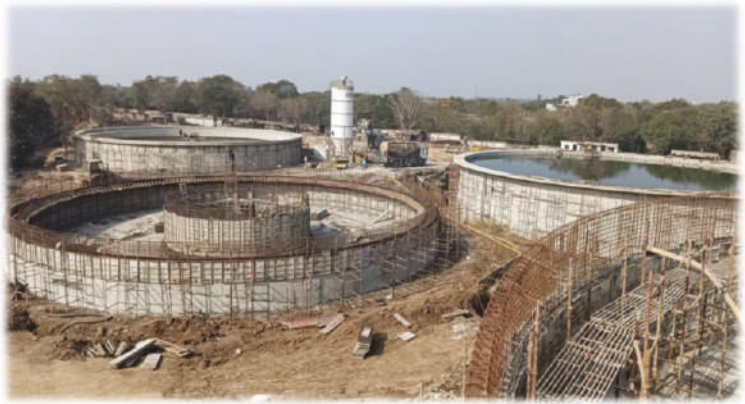
10 MLD CETP AT ANKELSHWAR
